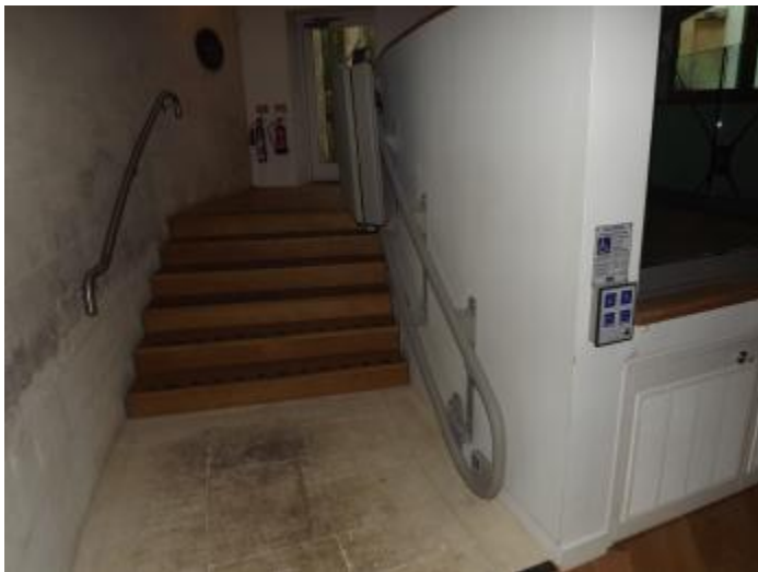
Platform lift into stables area
